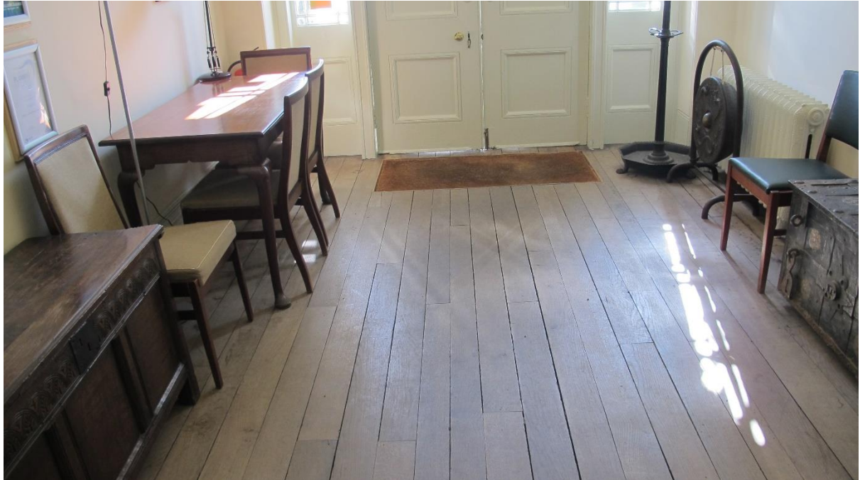
Figure 7. Entrance Hall of Parke with wood re-used from Higher Crownley. Frances Billinge 2018. By kind permission of DNPA.
